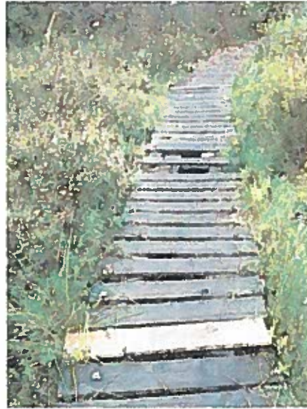
PHOTO: Former Bog Boardwalk
